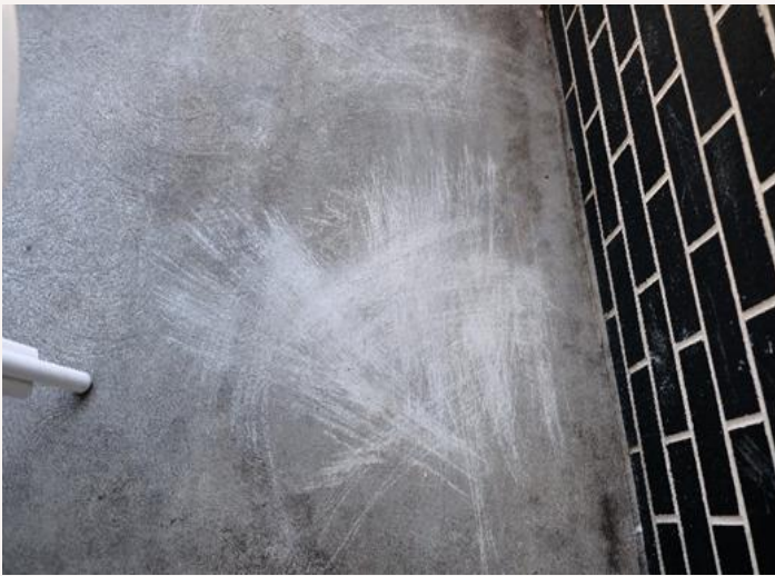
Damage to concrete consistent with sharpening of metal objects
