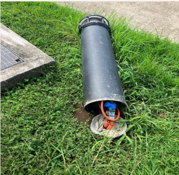
Pathway lighting with exposed wires
